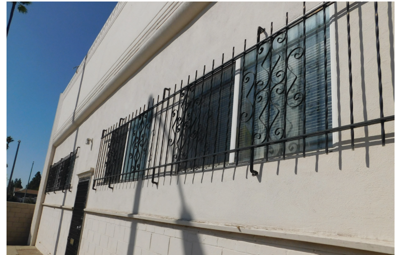
Example of exterior security bars (Prohibited treatment)
