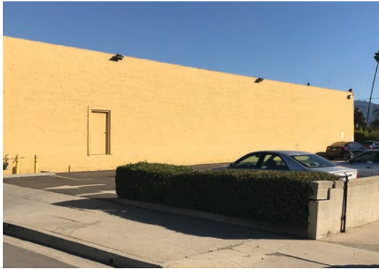
Example of a blank and windowless ground floor wall (Prohibited)
