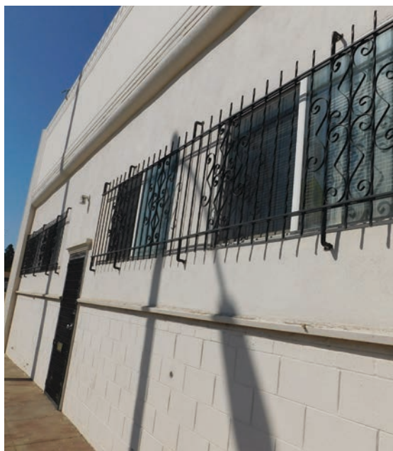
Example of exterior security bars (Prohibited)
